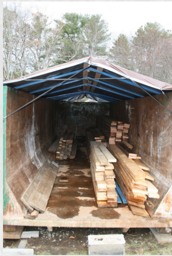
Lumber salvaged from the deconstruction of the house was collected in a 30 yard container to keep it dry, then donated to EcoBuilding Bargains.
