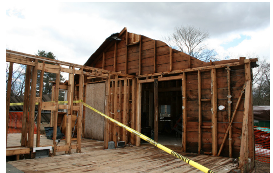
Careful deconstruction of two houses on the property ensured conservation of reusable materials.
